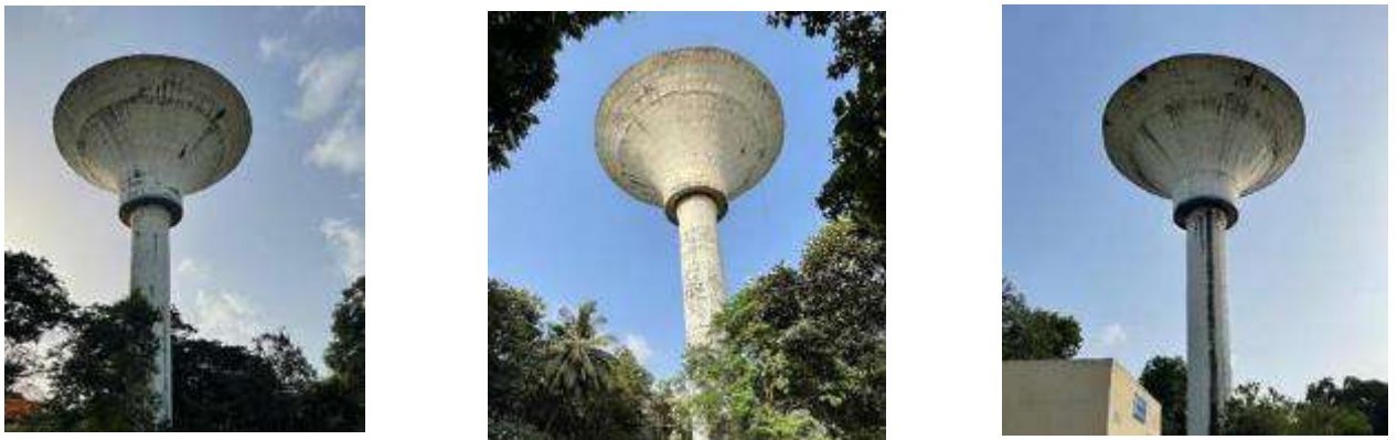
Figure 67 Three ESR of 0.35 MLD capacity each in JNPA township area
