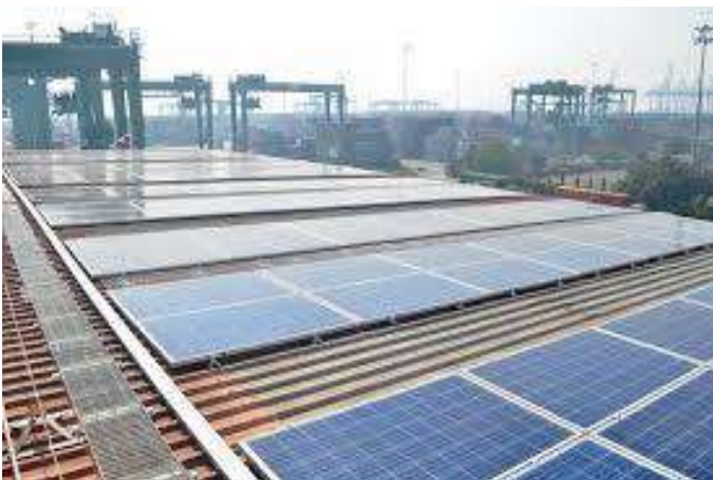
Solar Panels at JNPA
